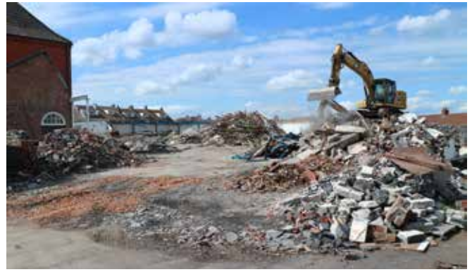
The main factory building was pile of rubble by early May
